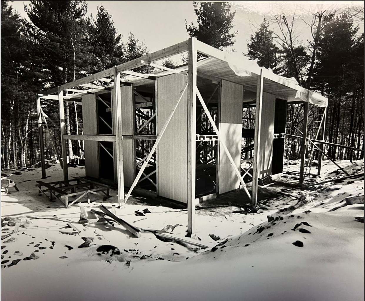
Figure 8. The System House, 128 Chichester Road, during construction (Collections of the New Canaan Historical Society).
